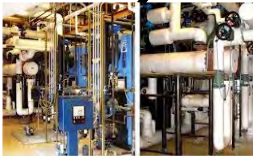
CENTRAL PLANT Natural Gas Boilers
