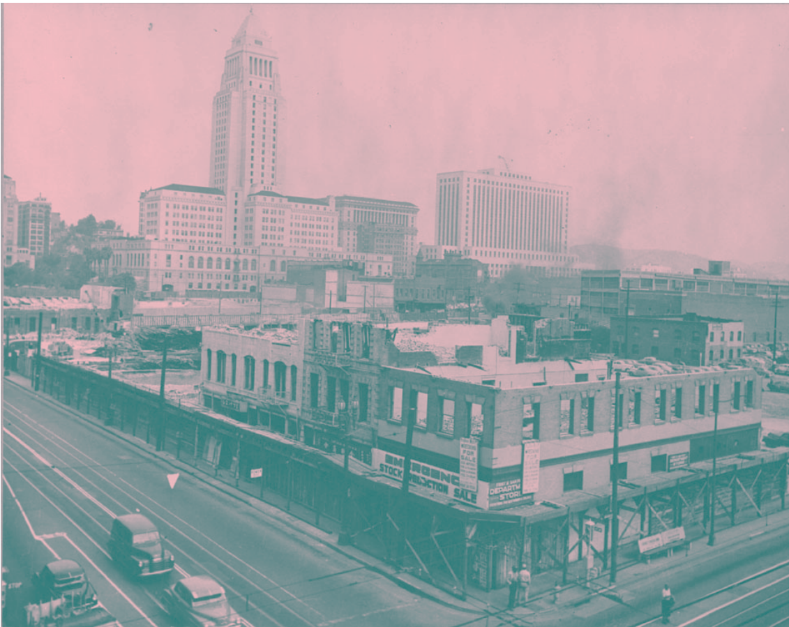
Figure 10. Demolition of Little Tokyo on the north side of First St, between Los Angeles St to San Pedro St, to make way for the LAPD's Parker Center.
